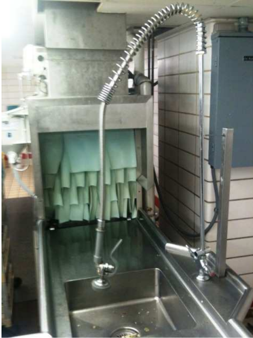
Figure1: Existing PRSV: T & S Bras B-0107-M, 1.42 gpm at 60psi
