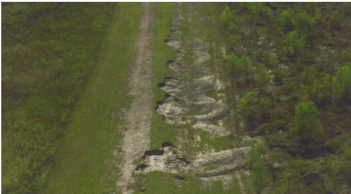
A-2. Example of overtopping-induced protected-side erosion on levee (IPET, 2007).
