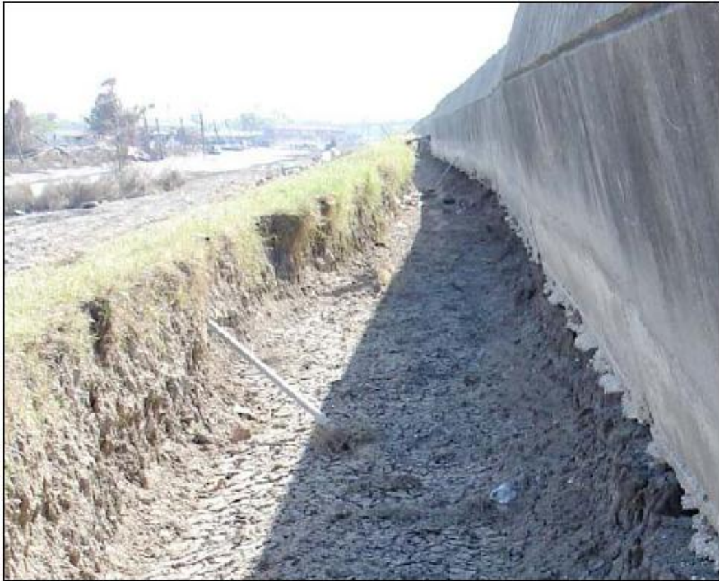
A-3. Backside floodwall erosion and tilting due to overtopping (IPET, 2007).
