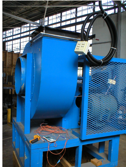
Figure 26: Motor and fan enclosure. An adjustable damper is located at the discharge of the fan (at the top).
