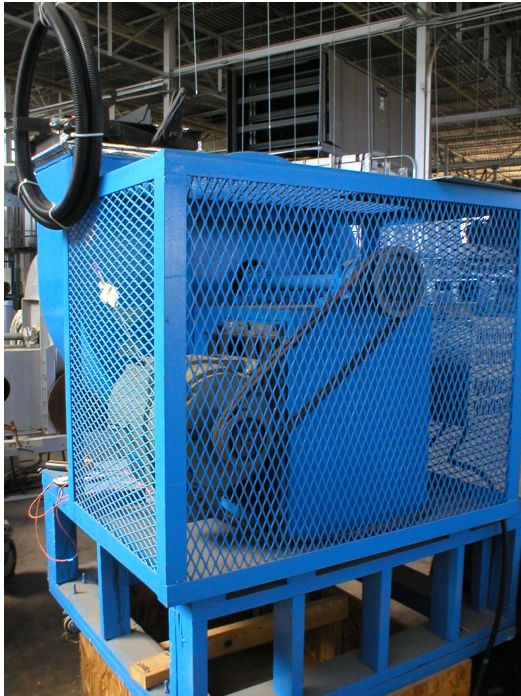
Figure 25: Motor #1 surrounded by expanded metal.
