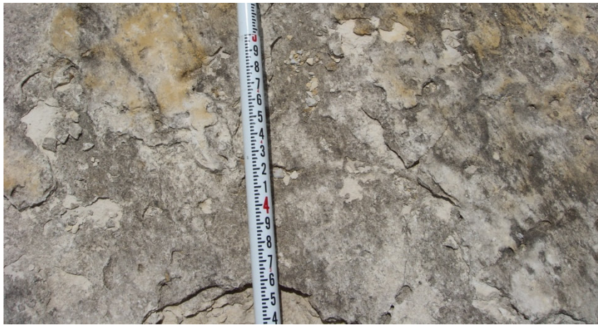
Figure 29. Rock unit 2-4. Unit 2-4 is a packstone that is 0.55 m (1.8 ft) thick. Weathering of the surface causes the rock to break into laminar sheets.
