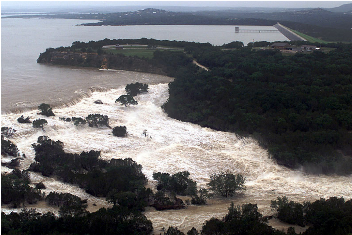
Figure 5. Photo showing flood waters overtopping the spillway ( http://www.cceo.org/FloodPics/index.htm , 2002). Canyon Lake Dam is seen in background. Comal County Engineers Office.
