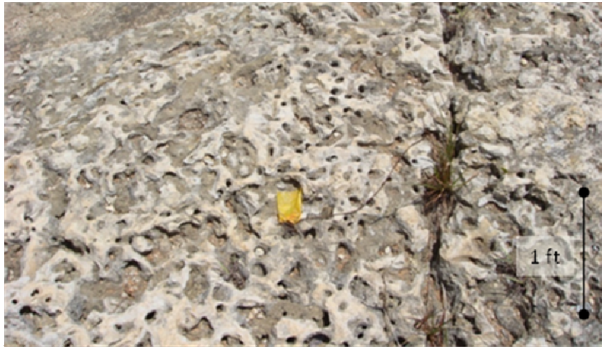
Figure 28. Rock unit 2-3. Unit 2-3 is a grainstone that is 0.85 m (2.8 ft) thick. Fracture density is low; at least seven ft (2.13 m) separate the larger surface fractures.
