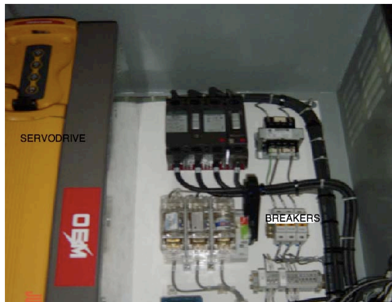
Figure A8. Breakers and Ser Dvdrive for Ladder and Cradle Control
