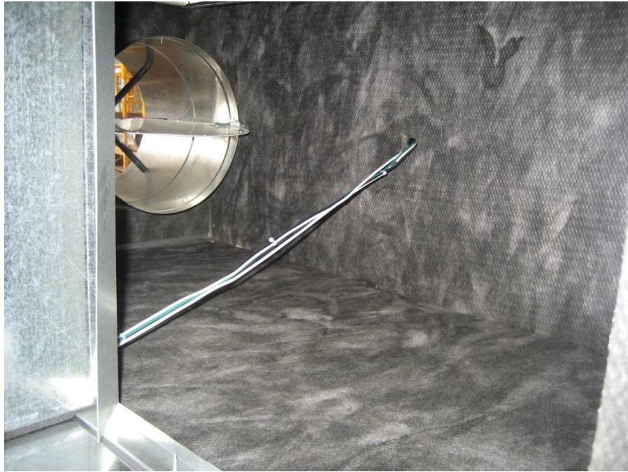
Figure 6-9: Cable Bundle Through Primary Air Stream for ECM_P12A
