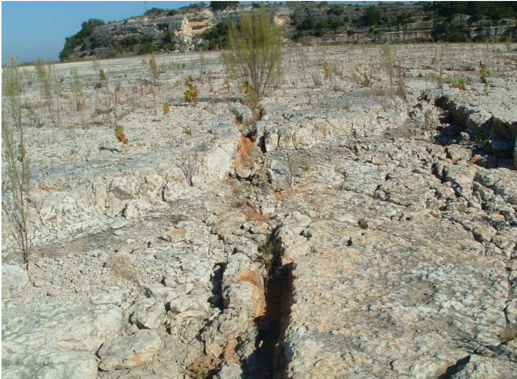
Figure 1.5. Shown here are joints widened by carbonate dissolution within the Glen Rose formation, Canyon Lake spillway, Canyon Lake, TX. The fracture, joint and fault patterns within a single rock unit typically trend parallel to each other.
