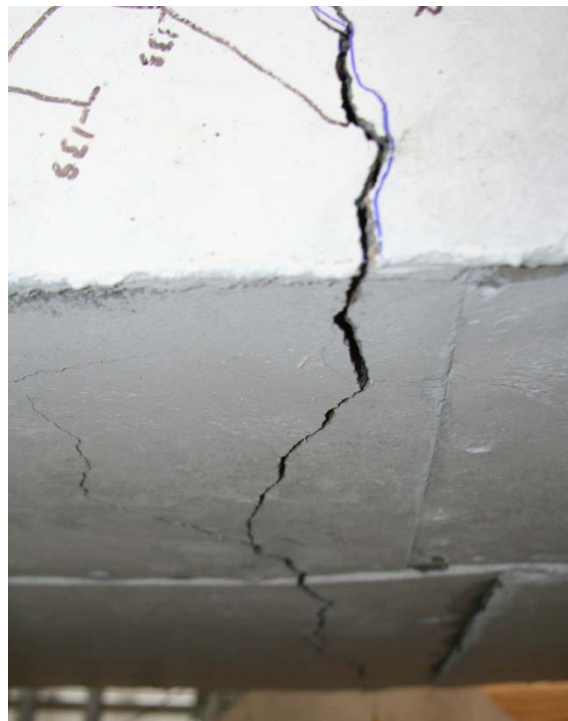
Figure 5-21 Tensile Crack at the Splice End on the Bottom
