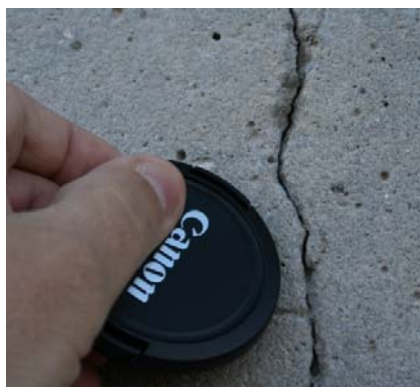
(b) Close-up of Crack
