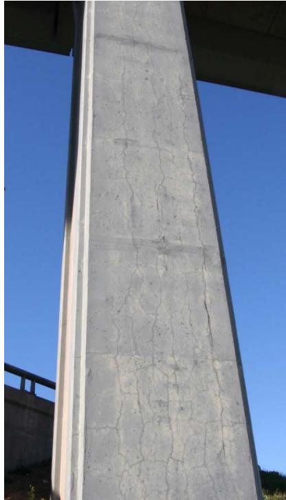
(a) Column with ASR Cracking
