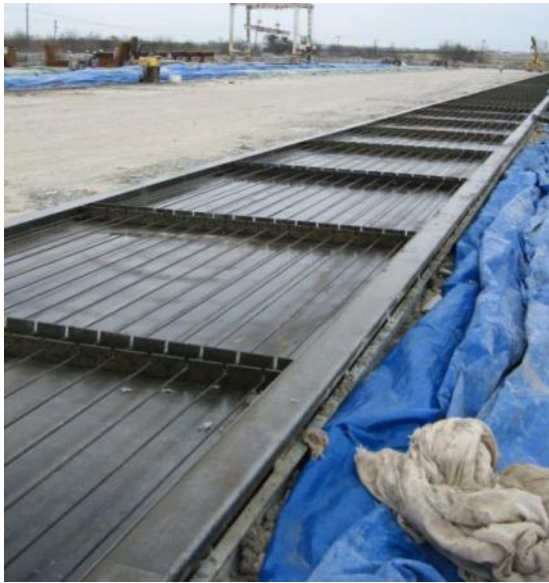
a) Long-line prestressing bed
