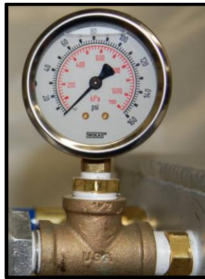
Fig. 2.14 Pneumatic motor input air pressure gauge
