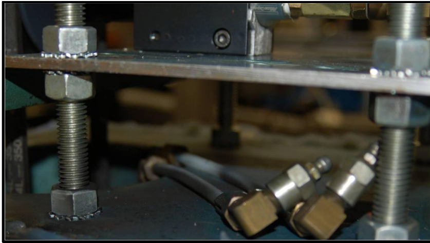
Fig. 2.7 Fan-shaft bearing grease lines
