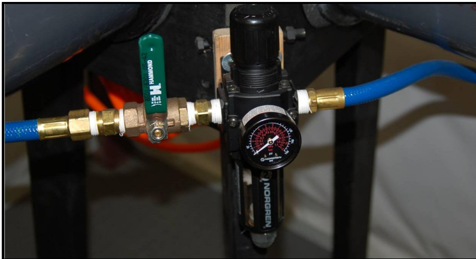
Fig. 2.16 Pneumatic motor regulator/filter assembly
