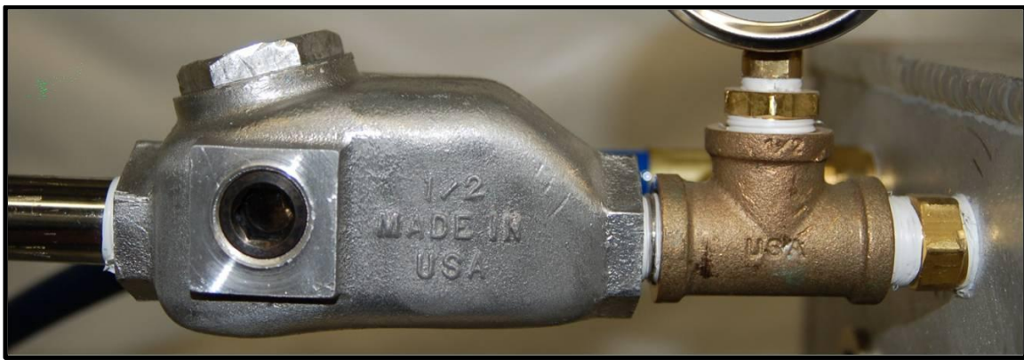
Fig. 2.12 Inline air lubricator
