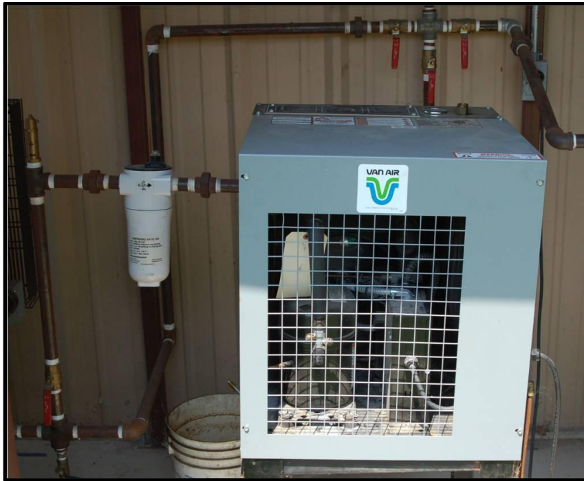
Fig. 2.21 Refrigerated compressed air dryer
