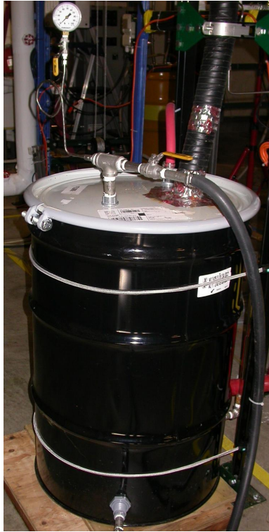
Fig. 4.7.: The steam-water outlet hose connected to the blowdown tank.
