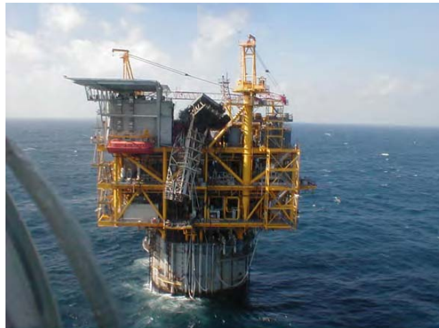
Fig 1-1 Side View of Medusa Platform after Hurricane Ivan (Murphy Exploration & Production Company, 2006)
