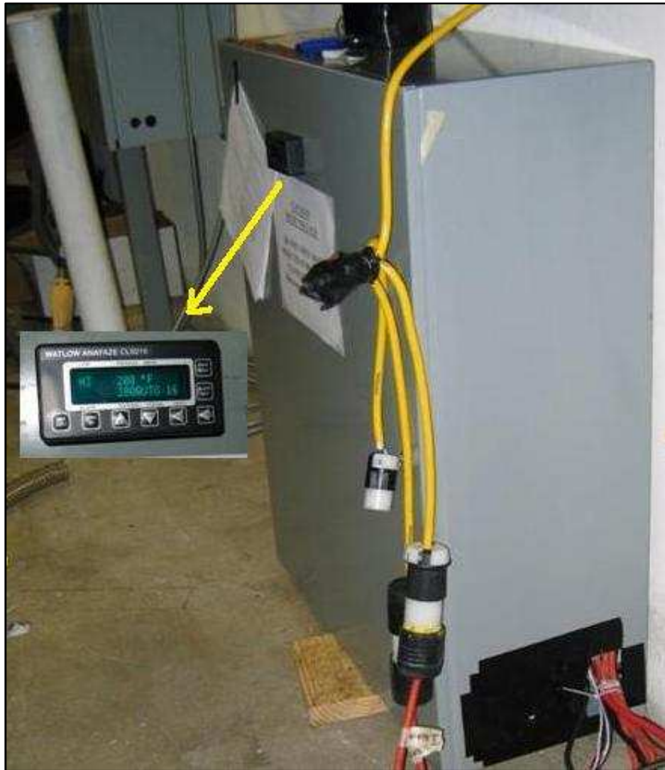
Figure 6-9 Heater controller cabinet and the controller (inset)
