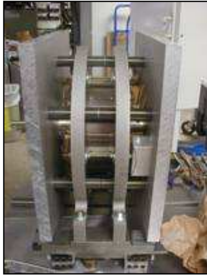
Figure 3-13 Stator and support ring alignment
