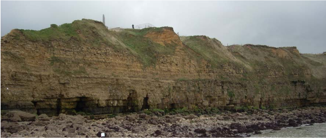
Figure 1.4. Basal wave-cut caverns at the western side of the point under the observation post.
