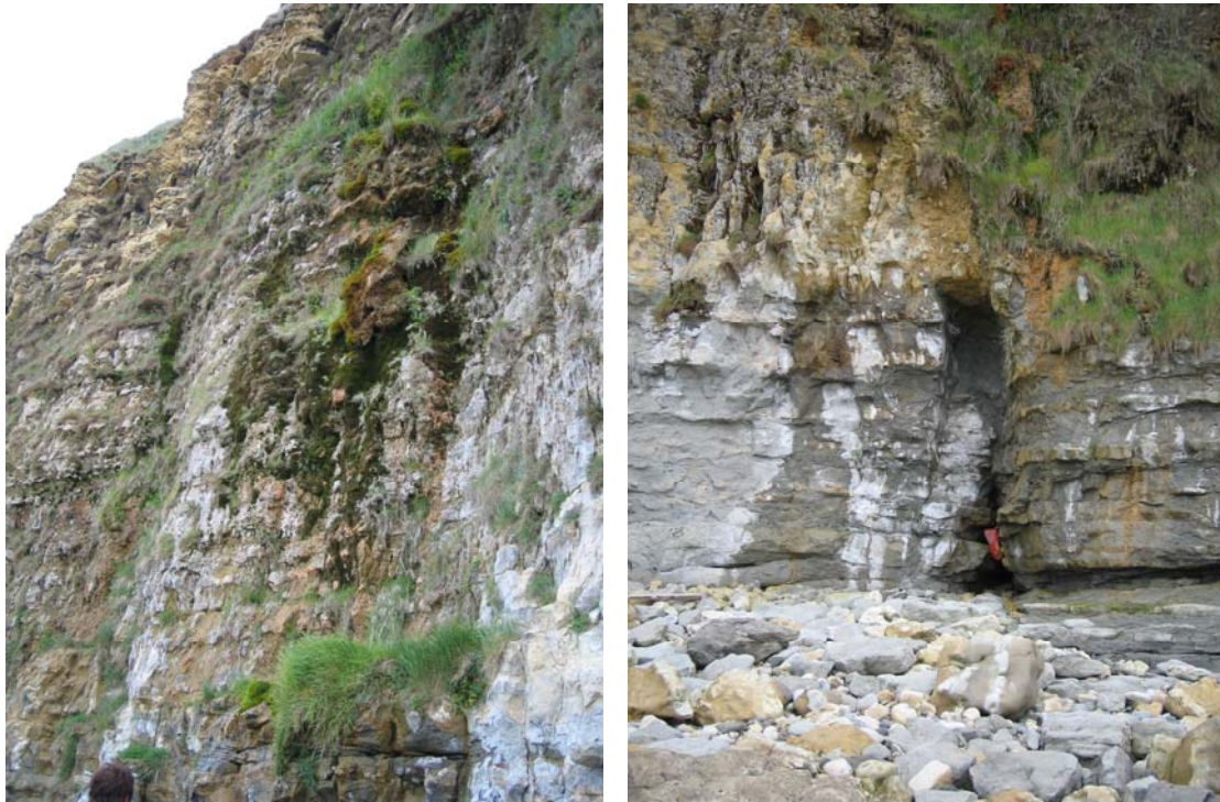
Figure 1.5. Groundwater cliff seepage.
