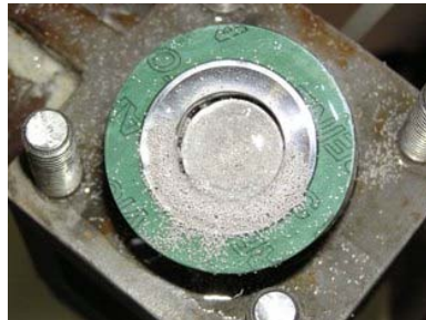
Fig. 4.10- Proppant particles prevent the valves from fully closing.
