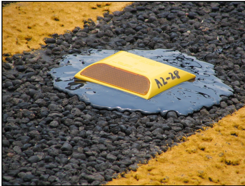
FIGURE 1 Typical non-snowplowable RRPM.
