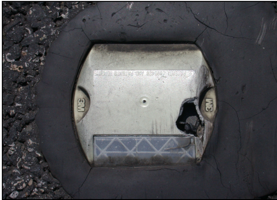
FIGURE 8 A common RRPM damage type.
