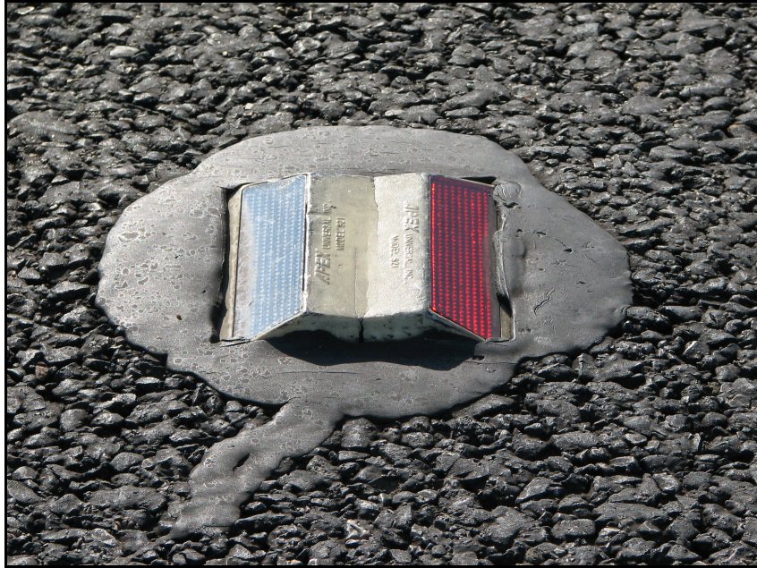
FIGURE 9 A typical damage type for RRPMs on flexible pavement.
