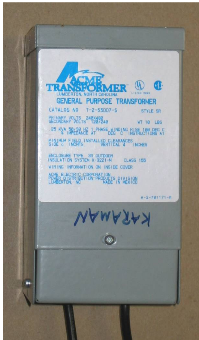
Figure 3.9 ACME step-up transformer used to increase the voltage supplied to heaters.
