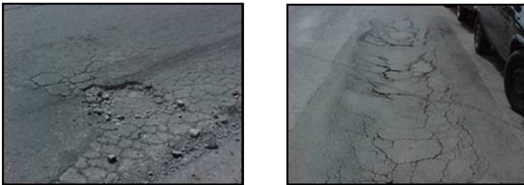
Figure 2.9. Detrimental effect of water in the severity of pothole (left) and patch deterioration (right)
