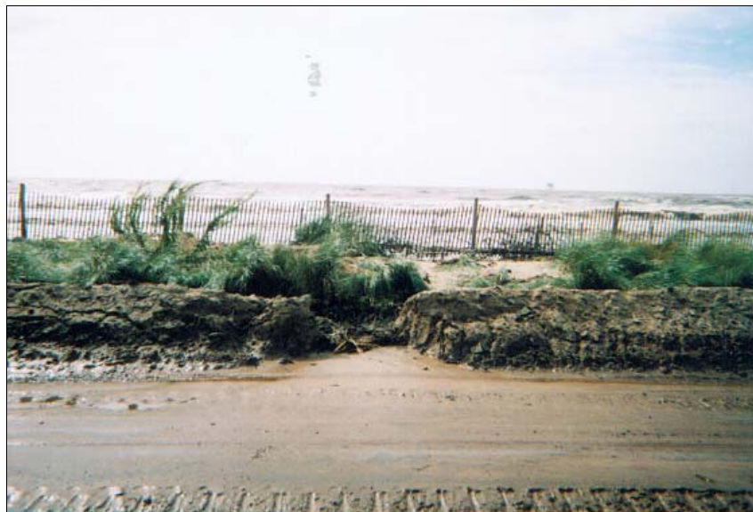
Fig. 3.8. Berm destruction by overwash prior to the landfall of tropical storm Ivan in the survey area on September 23, 2004.
