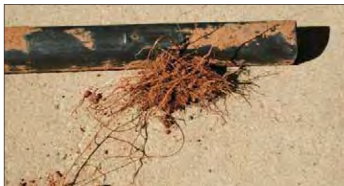
Figure 5. Roots penetrating a drip emitter.
