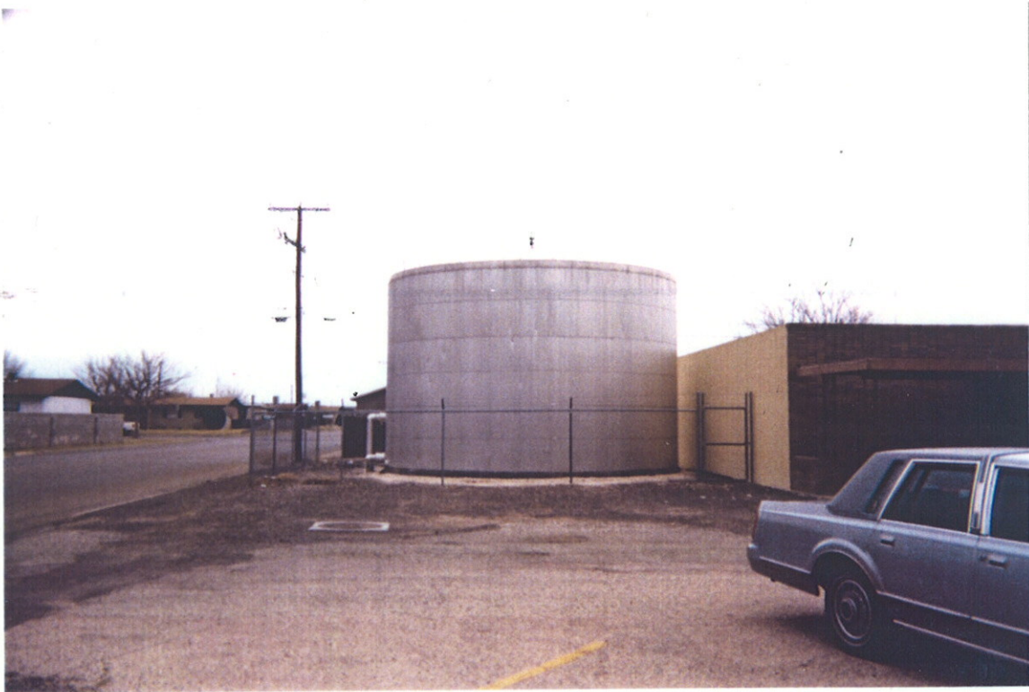
Chilled Water Storage Tanks
