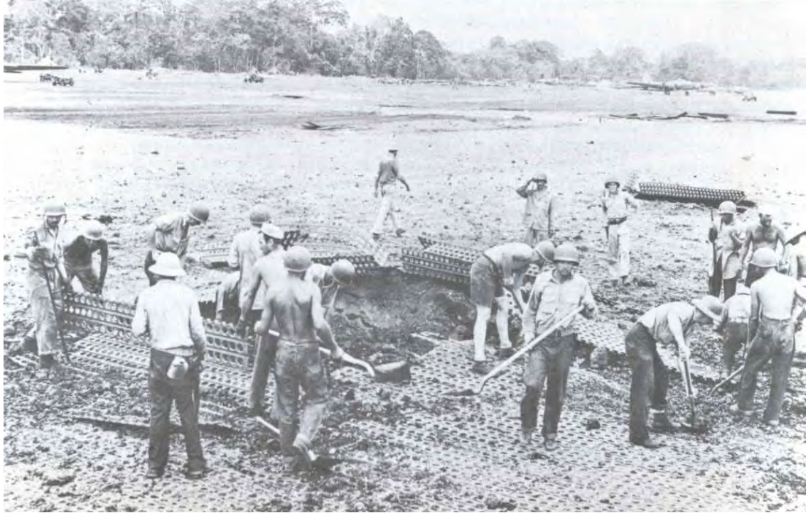
Ground crews were called on to rebuild the airfield after every Japanese bombing attack. Note the steel mesh that was laid down on the surface to improve the usefulness of Henderson.
