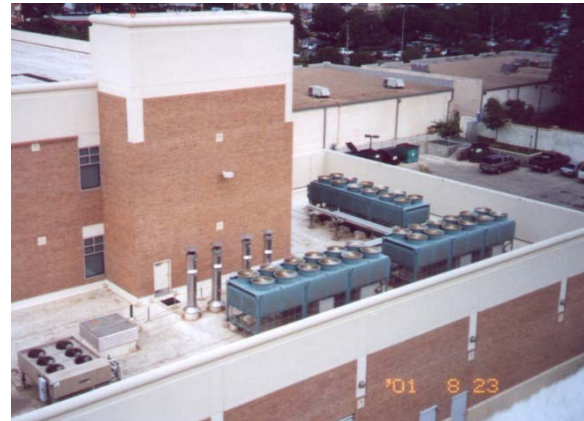
Figure 14. Hospital Chiller Installations
