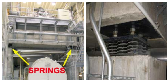
Figure 8. Turbine Pedestal Base with Spring Isolators
