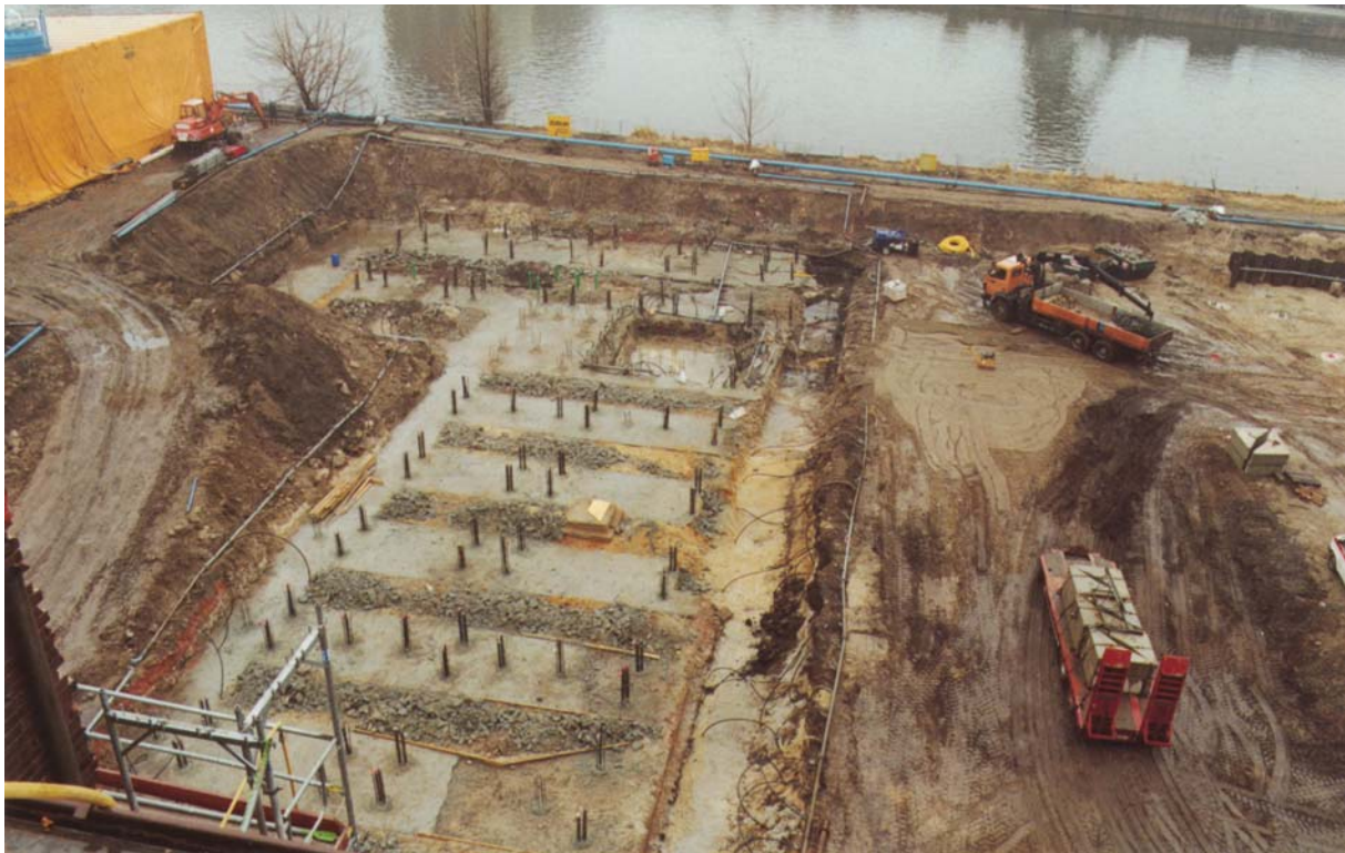
Figure 1: Energy piles under construction: pile pattern of an office building near Spree riverside, Berlin
