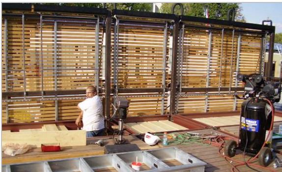
Figure 26. Solar Thermal Collector Manifold.
