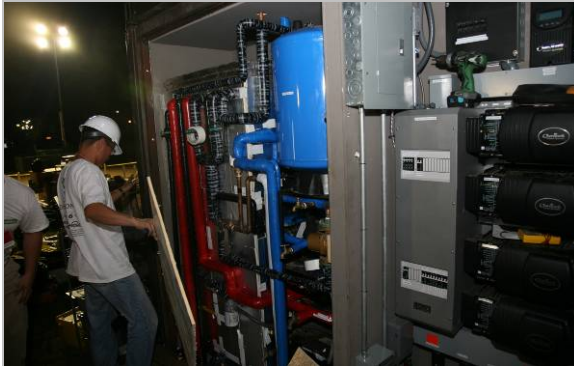
Figure 25. Components of Solar Thermal System.
