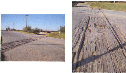
Bell St Main: 21 481 D – VERY BAD
