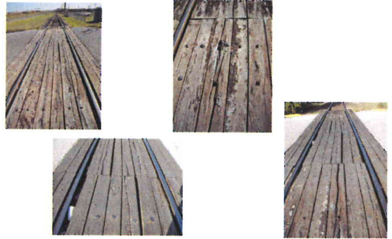
N. Pope St: 21 512 P – POOR
