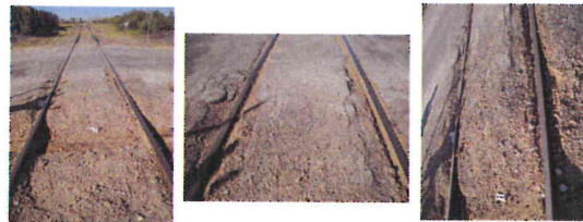
Upton St: 18 741 R - POOR
