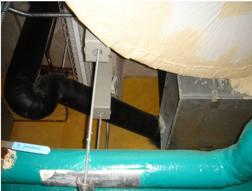
Figure 106: Installation of a Portable Logger to Measure the Return Air Temperature of an AHU on the 5th Floor
