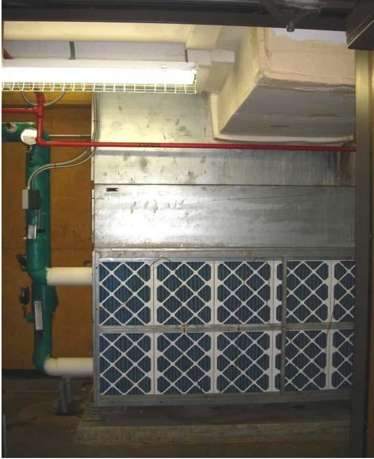
Figure 105: Air Handling Unit in the 5th Floor of the John Connally Building
