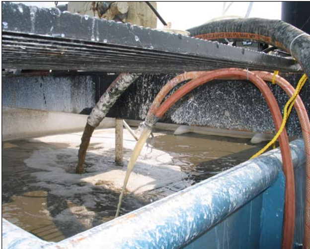
Figure 8: Mixing tank with chemical additions.
