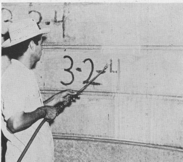
Figure 12. A good clean-up campaign was necessary for effective insect control. After the clean-up, a 2.5 percent methoxychlor spray was applied, to the point of runoff, to the inside walls, as shown here. A DDT spray was applied to the outside walls and to the soil near the bin, but was not used where it might contact the stored grain.
