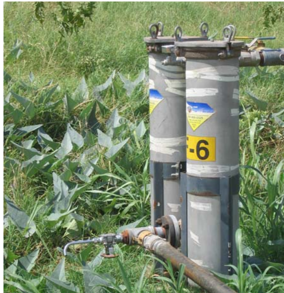
Fig. 7. The Final Filter and Port for Effluent Sampling
