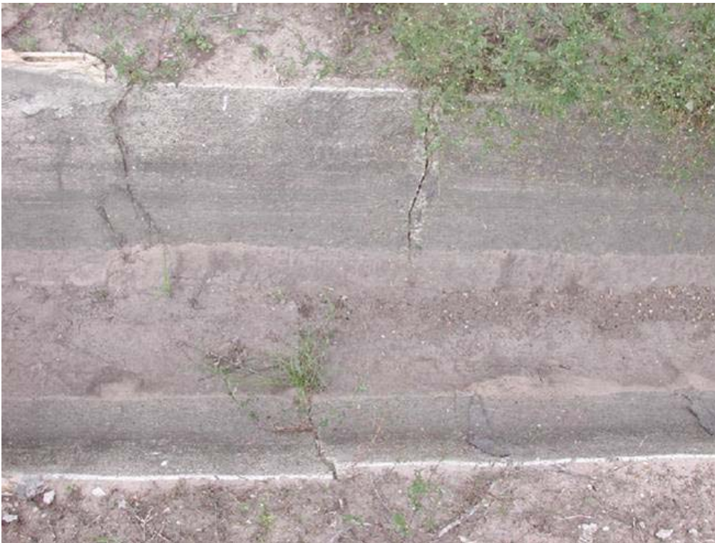
Figure 4. Example of pencil-sized cracks (C), 3 to 5 feet apart.
