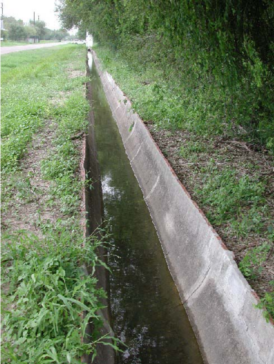
Figure 5. The white marks on the right side of this canal highlight pencil-size cracks (C) spaced over 10 feet apart.
