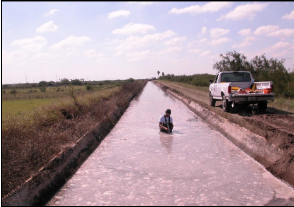
Figure 3. Photograph of the installation of a staff gauge in Test Segment 16HC2.
