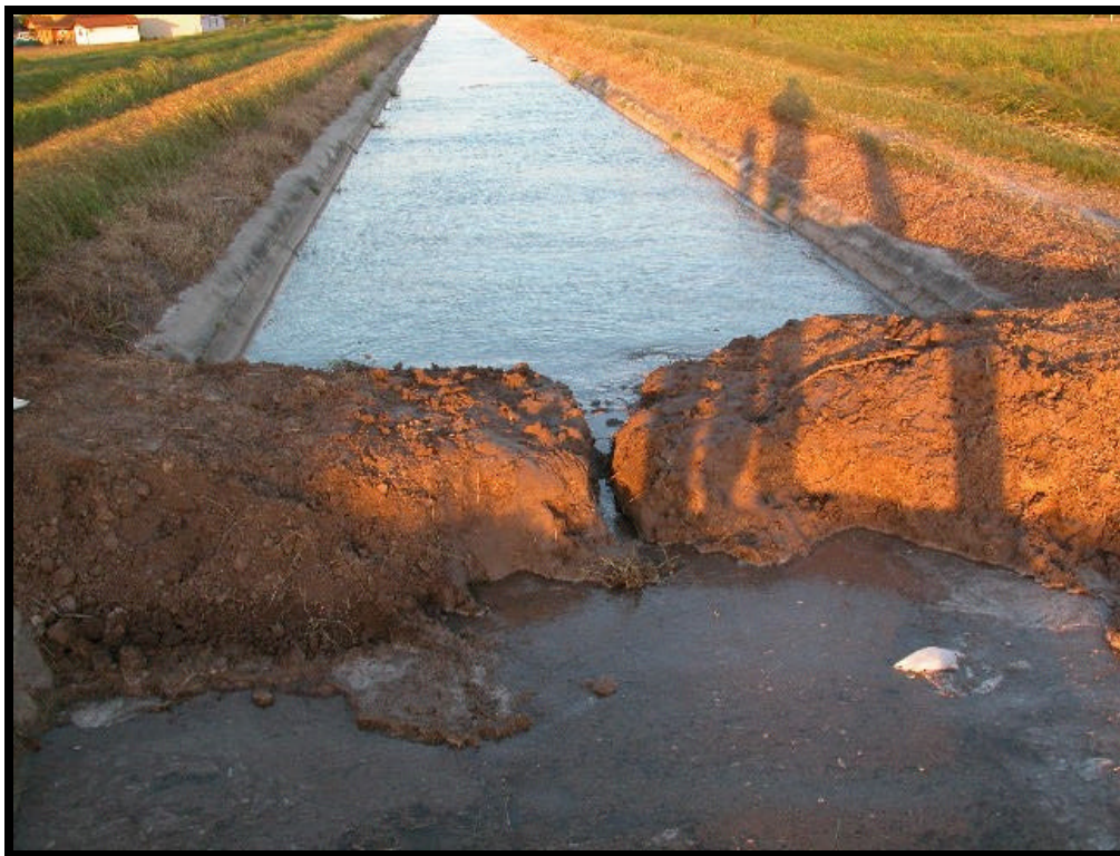
Figure 5. Photograph of damage to the dam between segments SJ10 and SJ11 that caused early termination of test.
