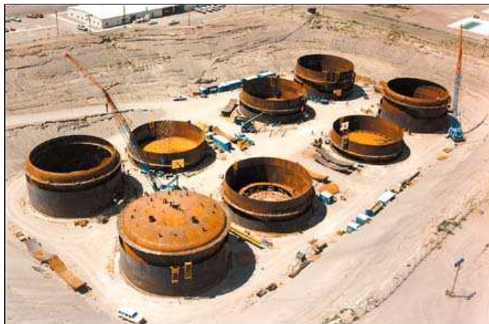
Figure 1.1. Waste tanks are made of steel and are 30 feet in diameter. Some are buried and capped with clay leaving only important access points exposed.
