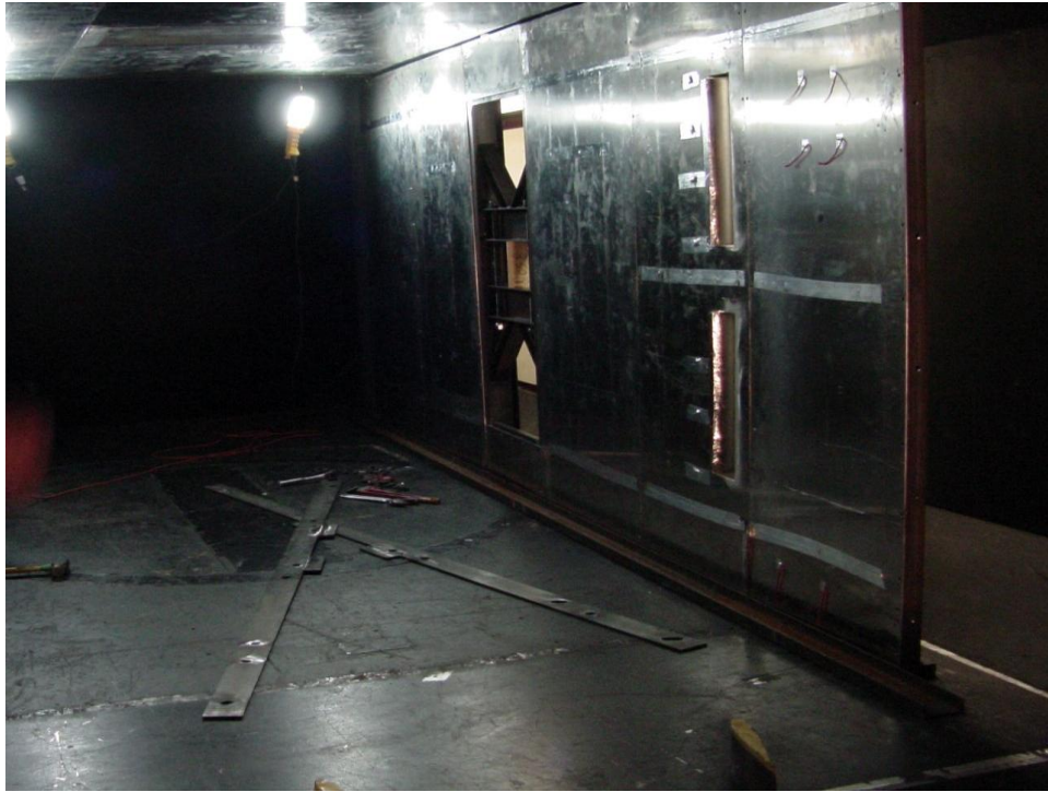
Figure B-6 Installation of right side wall with the C-channel for alignment
