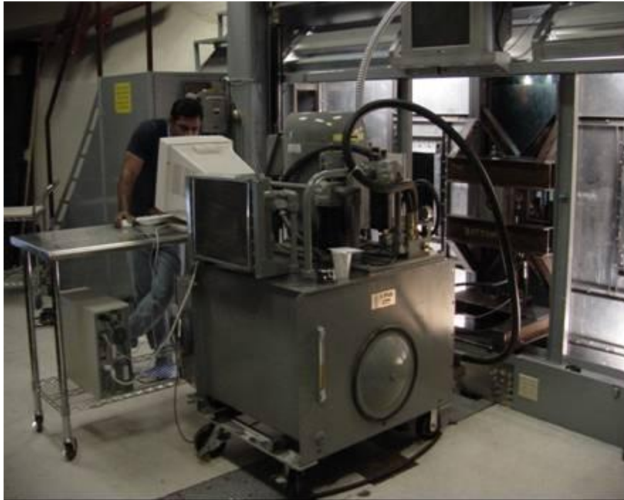
Figure 51: Hydraulic drive system reservoir
