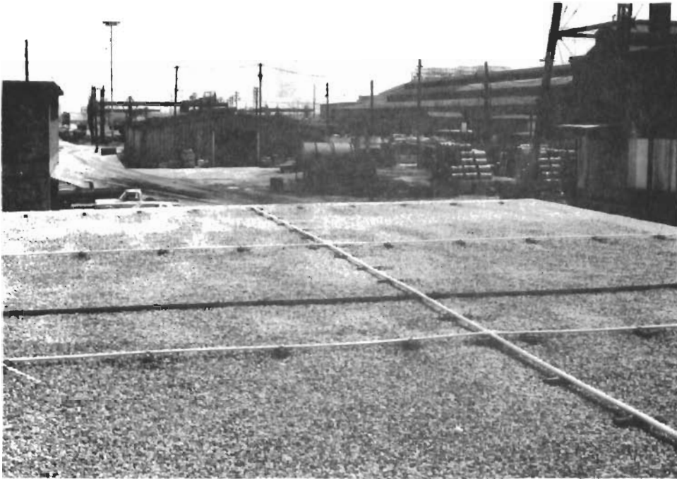
Roof spray grid at the Armco Steel plant Engineering Office, Houston, Texas.
