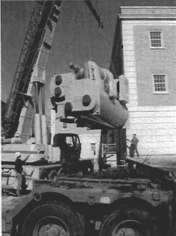
New 1200 ton chiller at the UNT power plant
