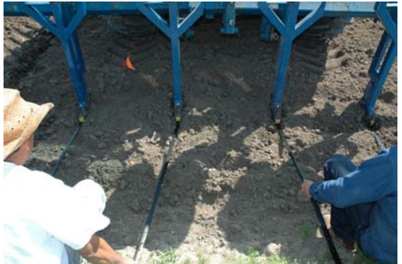
Tape being installed at a depth of 10", which allows for disking and plowing of fields without damage.
