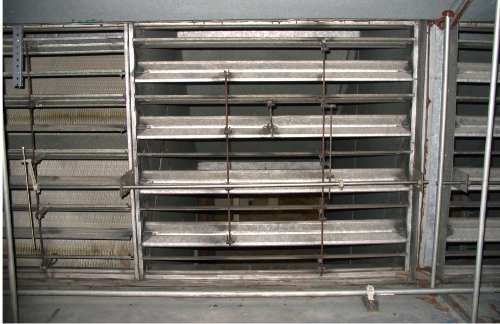
Figure 6. Heat Exchanger Dampers in New Configuration.
