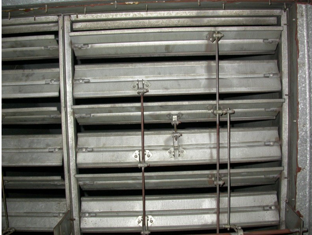
Figure 5. Heat Exchanger Dampers in Original Condition (Fully Open).
