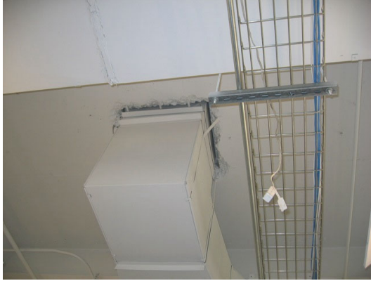
Figure 12. Potential Leakage Sites - Where Ducts Penetrate the Third Floor Ceiling
