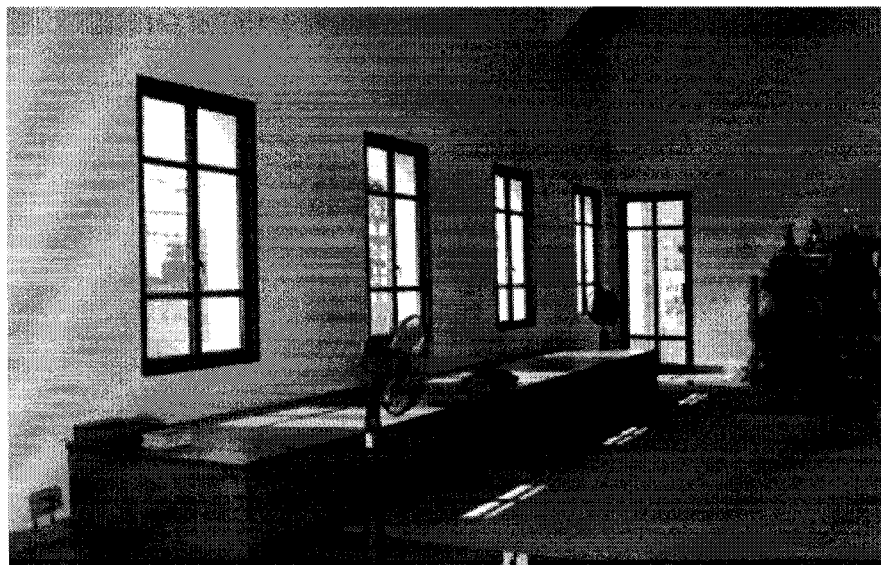
Figure A.7 Interior View of the New Temple Showing the Interior Wall at the South Side of the Building. This picture shows that the windows were not properly shaded from the direct sunlight. This caused the space to be hot for most of the year.
