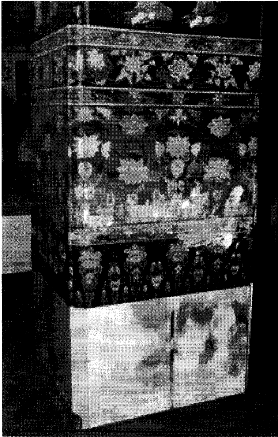
Figure A.4 Moisture Problem in the Old Temple. This picture shows a surface of an interior column where mold and mildew grew and destroyed wall paintings.
