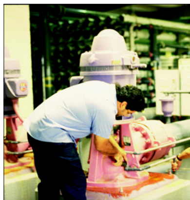
Figure 10. Purple pumps and pipes designate recycled wastewater at Harlingen Water Works wastewater treatment plant. After a stringent treatment regiment, wastewater is pumped to an adjacent bleach-and-dye plant.
