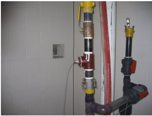
Figure 7.10 The soapstick dropping connection and 4" loop with the pressure gauge connection at the wellhead (9 th floor)
