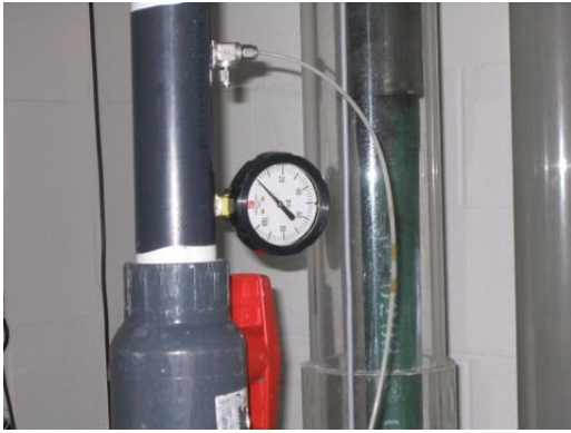
Figure 7.8 Pressure gauge and pressure transmitter connection at the 6 th floor to measure the pressure at the middle of the tower around Auger Tool
