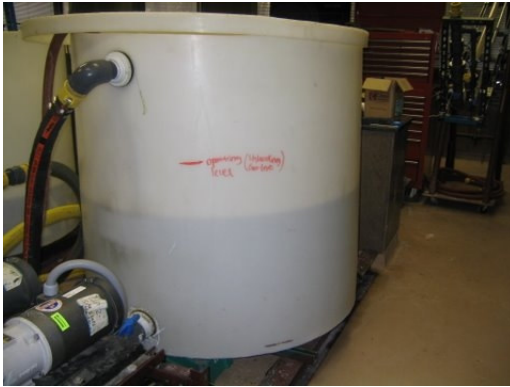
Figure 7.16 Covered tank used for water and foam storage during the test with water and foam
