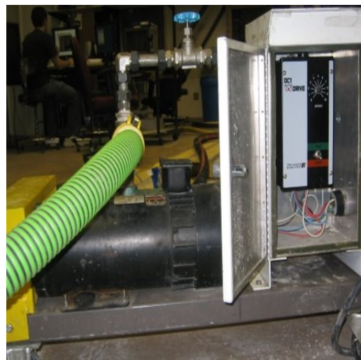
Figure 7.15 Variable frequency drive (VFD) controller to provide operability range with the pump
