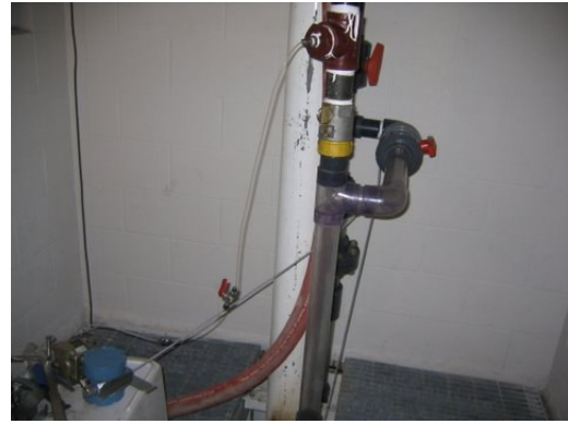
Figure 7.9 The wellhead connections at the 9 th floor with the wellhead loop and pressure transmitter
