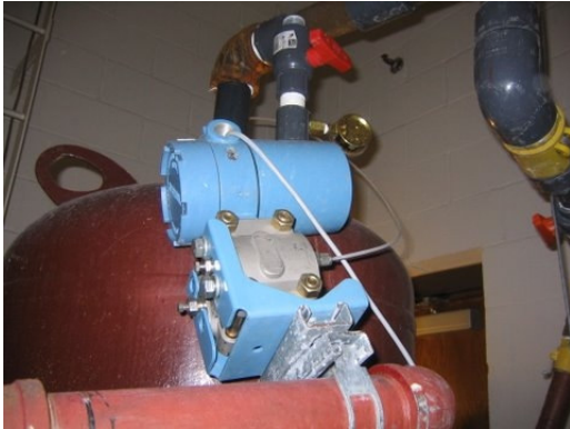
Figure 7.4 Pressure transducer in the wellbore with the surge vessel (3 rd floor)
