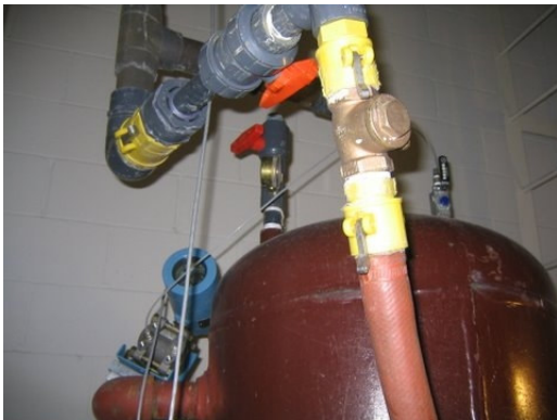
Figure 7.6 The air and water connection meeting at the wellbore (3 rd floor)
