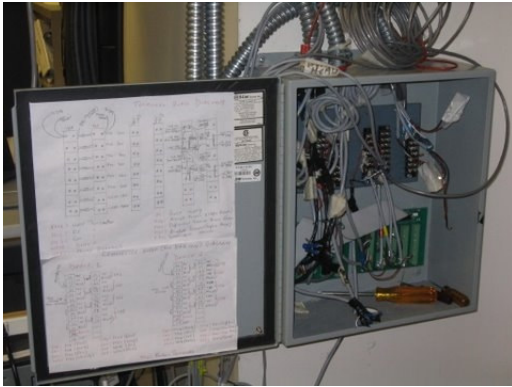
Figure 7.12 Junction box with instructions
