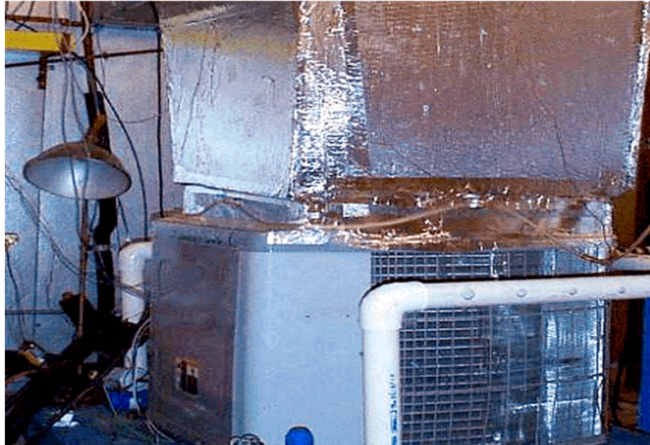
Figure 3.23 The externally manifolded pressure taps used to measure the static pressure at the exit of the outdoor unit
