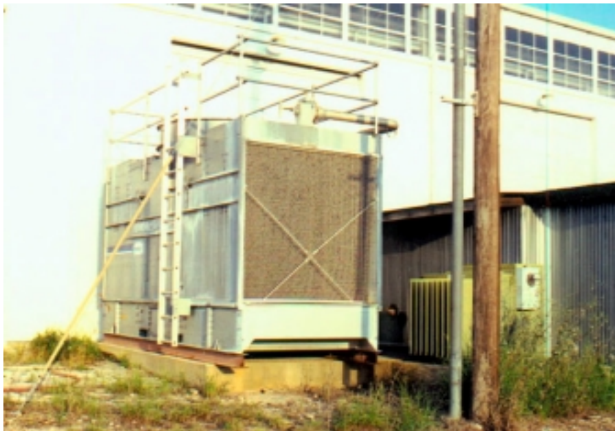
Figure 3.9 The cooling tower at the Energy Systems Laboratory
