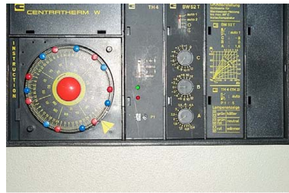
Measure 3: Adjustment of heating times to utilization: Switch off Sa + Su, postpone start of heating-up operation Mo – Fr from 2, 3 and 4 o'clock respectively to approx. 5 to 6 o'clock.
