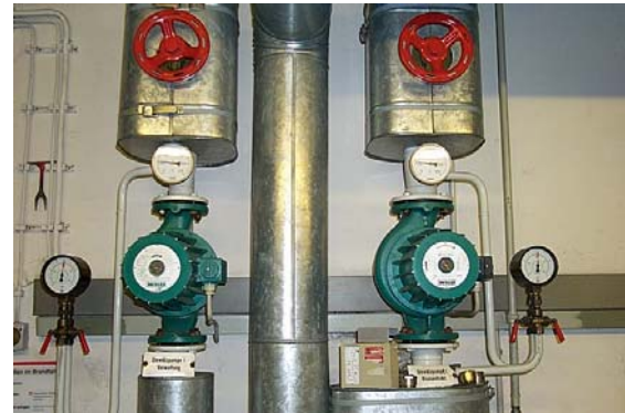
Measure 4: Pump operation on a trial basis with reduced power.
