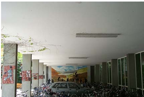
Measure 2: Insulation of the floor slab against ambient air. Comfort problems in relevant rooms.
