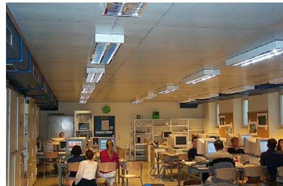
Measure 7 and 9: Ventilation installation computer room: Switch off ventilation completely if possible, windows are existing. (...) If fresh air operation necessary, stage 1 sufficient. Check ducts: supply air outlet barely perceptible, although air change of 3,600 m 3 /h is set.
