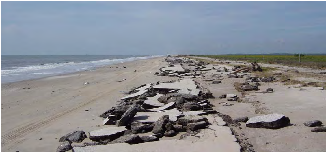
Fig. 8. Near CATT where road is destroyed, picture taken October 5, 2002.
