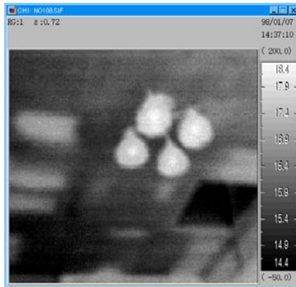
Figure 5 insulation defect at ceiling of living room
