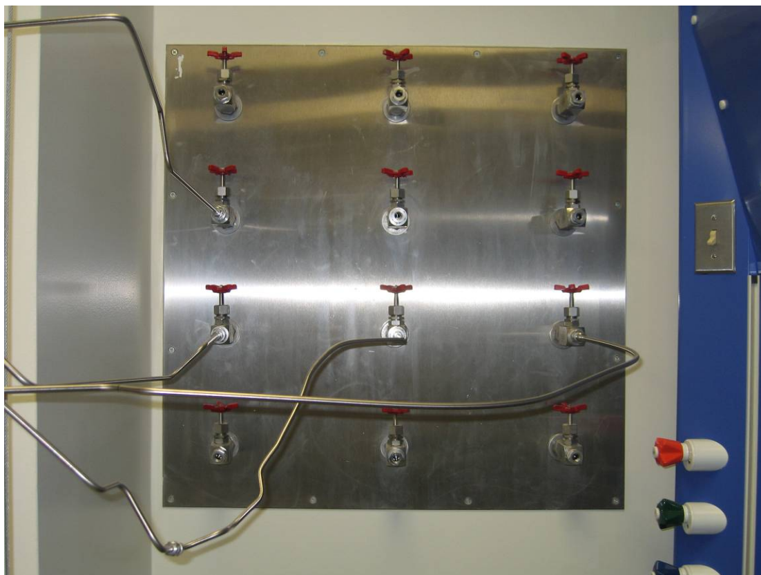
Fig. 4.8. Gas feed wall panel.
