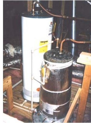
Figure 8. Solar heated tank
