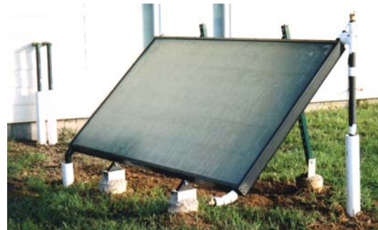
Figure 9. Hot water solar collector
