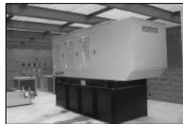
Figure 2. Typical Generator Set
